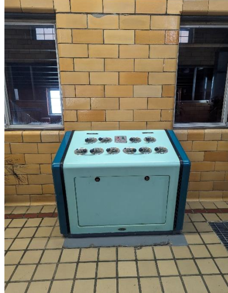
SOFTENER CONTROL CONSOLE
