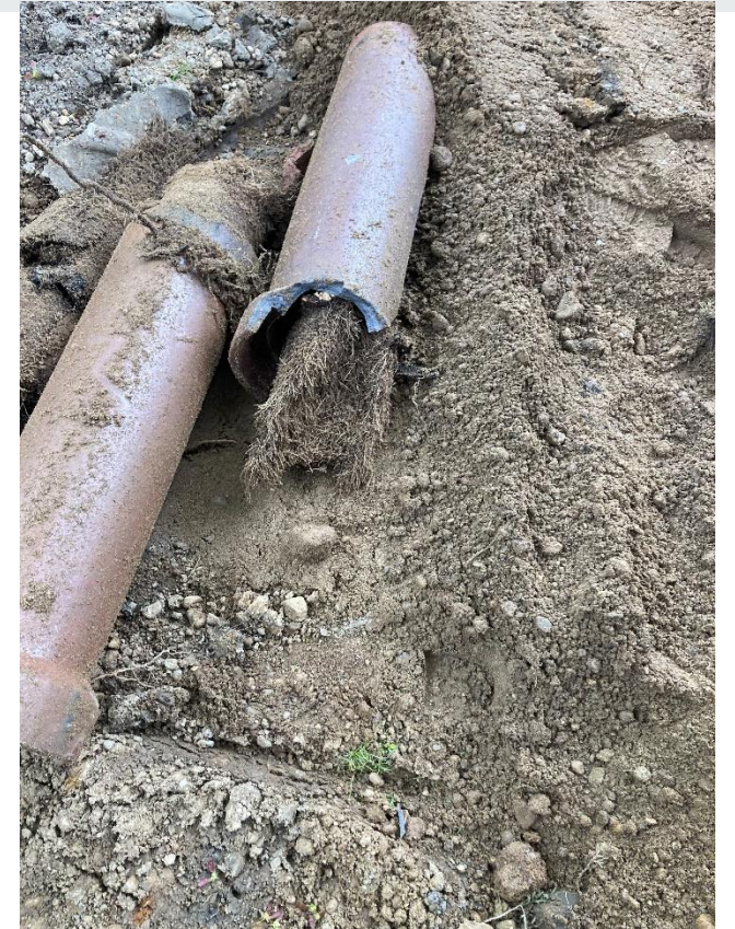
ROOTS IN SEWER LINES
