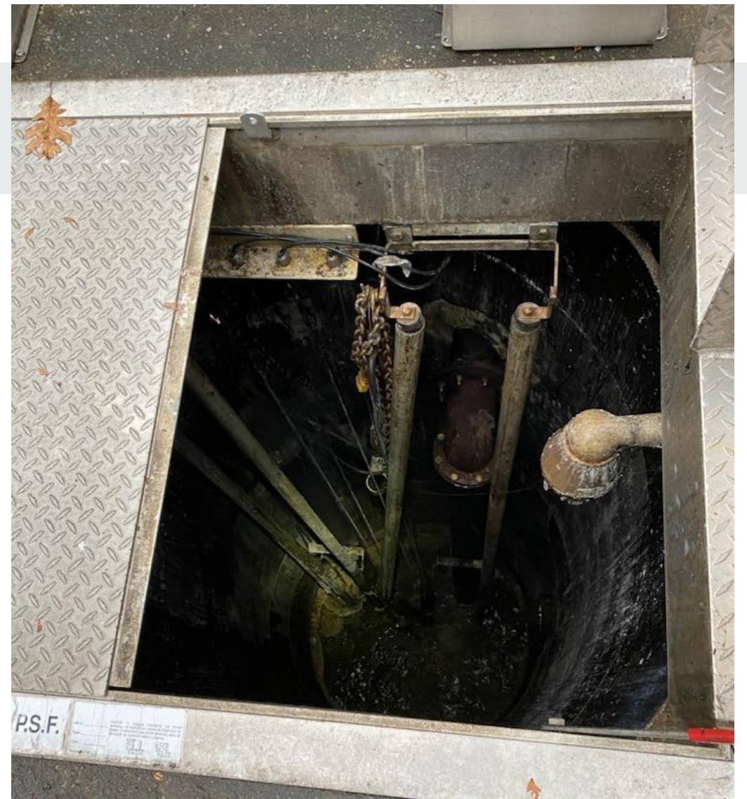
HIDDEN LAKES PUMP STATION
