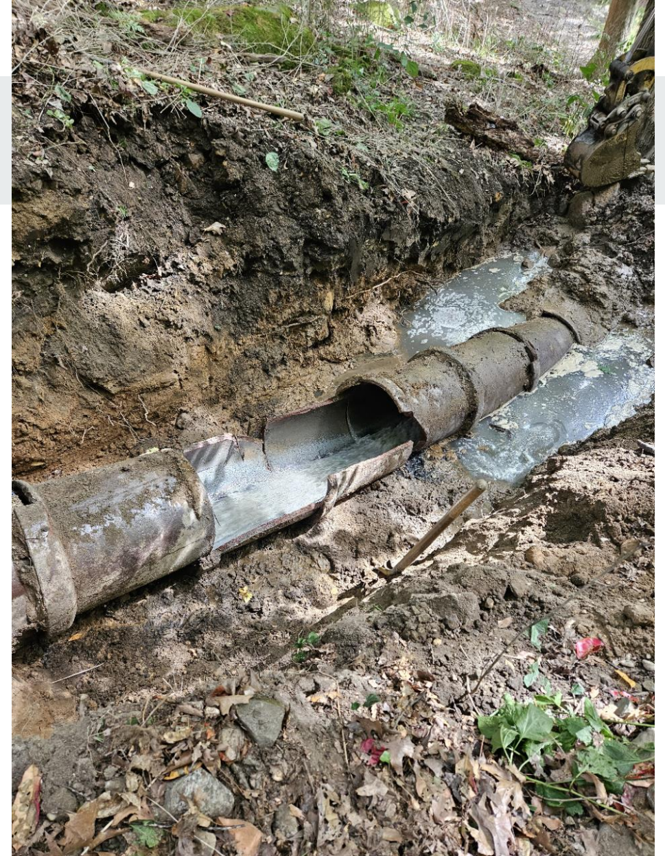
GORGE TRUNK SEWER BREAK
