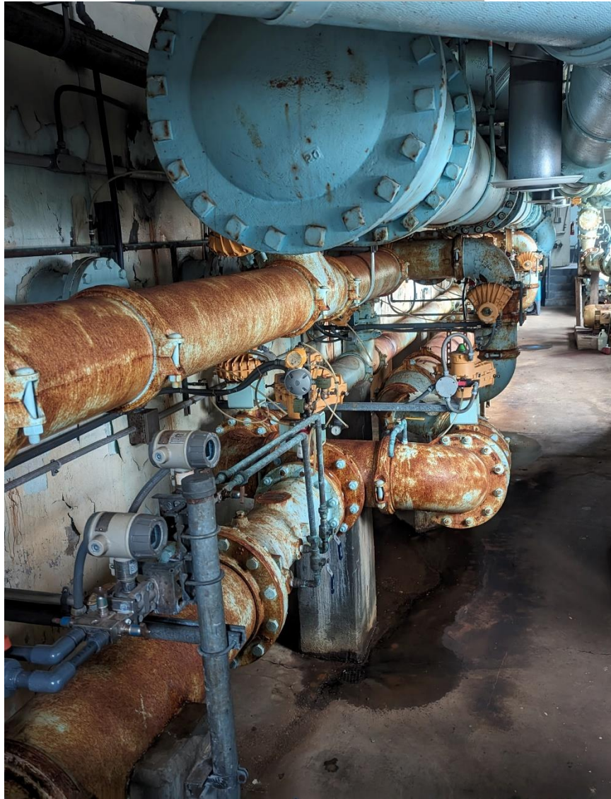
FILTER PIPING GALLERY AT WTP
