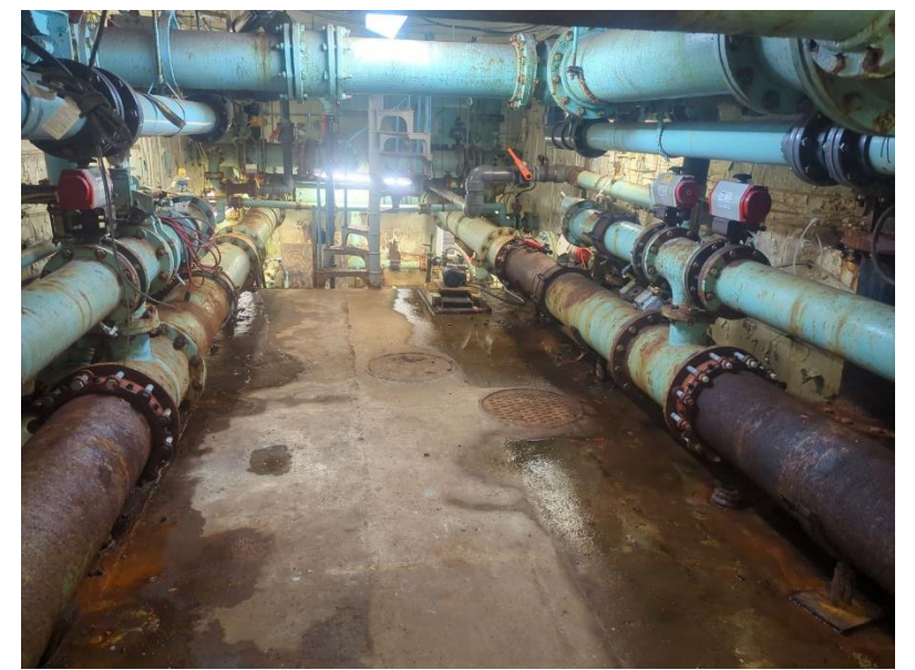
SOFTENER PIPING GALLERY TO BE REPLACED
