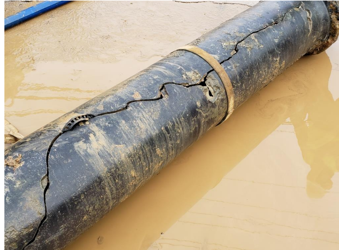
MAIN BREAK ON STATE ROAD = 2018
