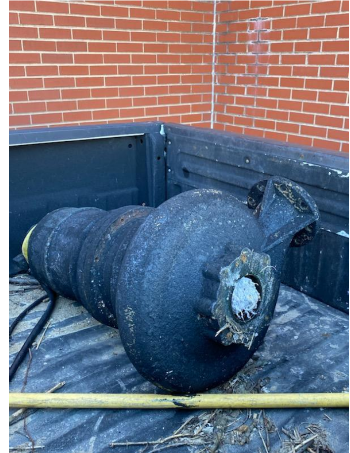
SEWER PUMP NEEDING REPAIR
