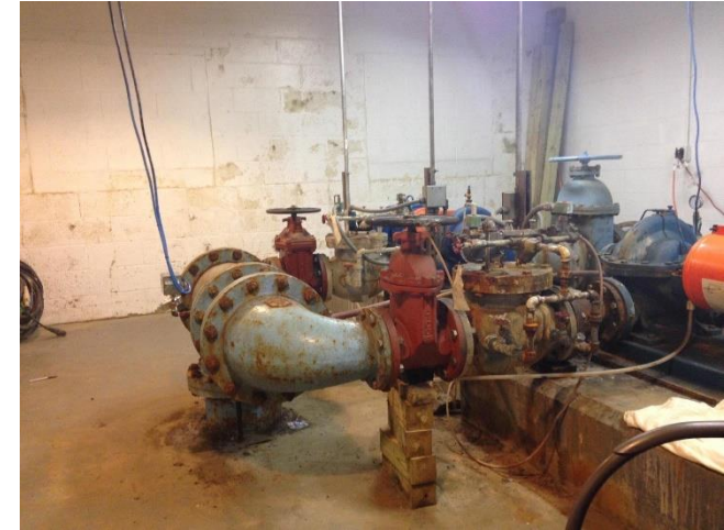
BAILEY ROAD BOOSTER PUMP STATION
