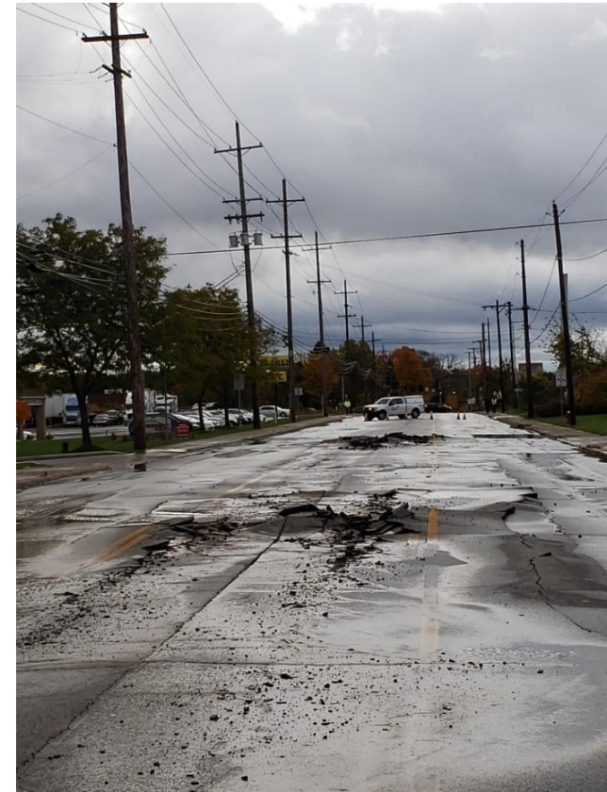
STATE ROAD WATER MAIN BREAK: NEW PAVEMENT RUINED
