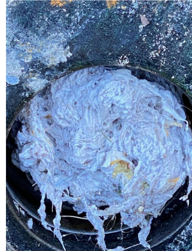
RAGS & "FLUSHABLE" WIPES IN PUMP
