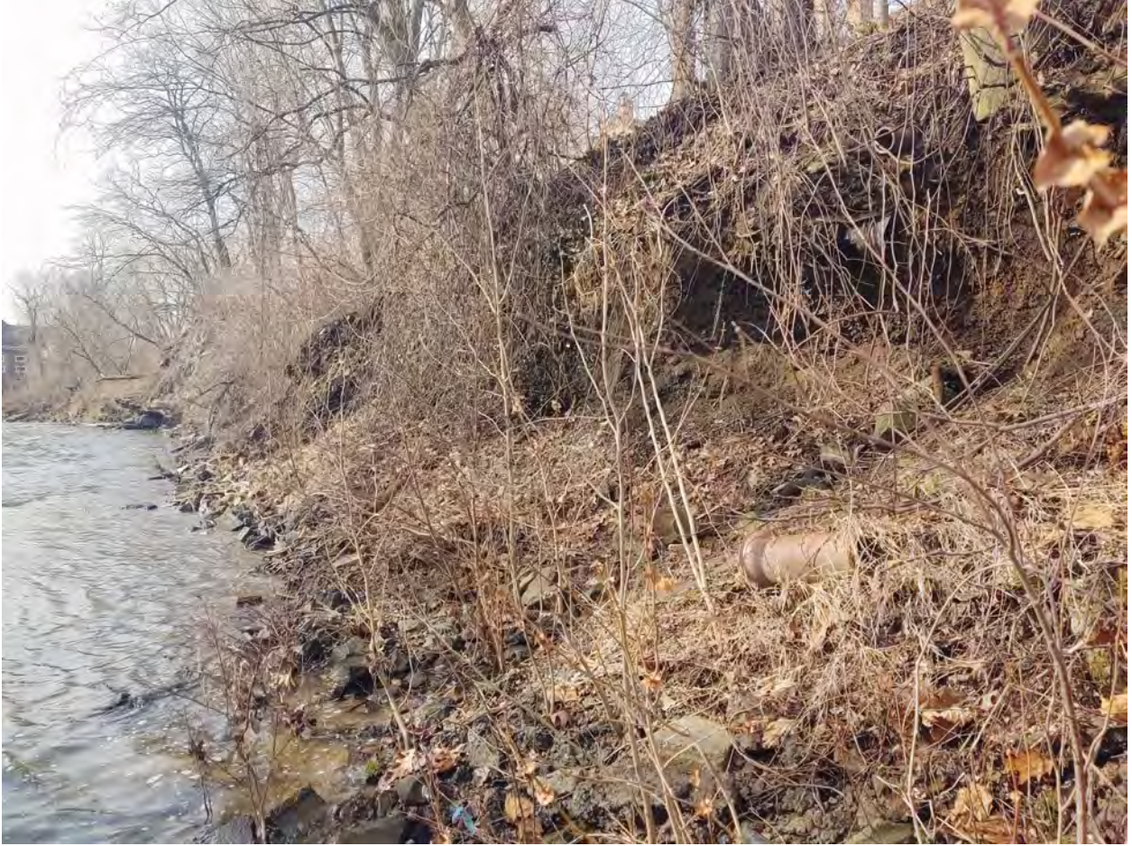
Photo 2. Upstream view of the erosion within the project site.
